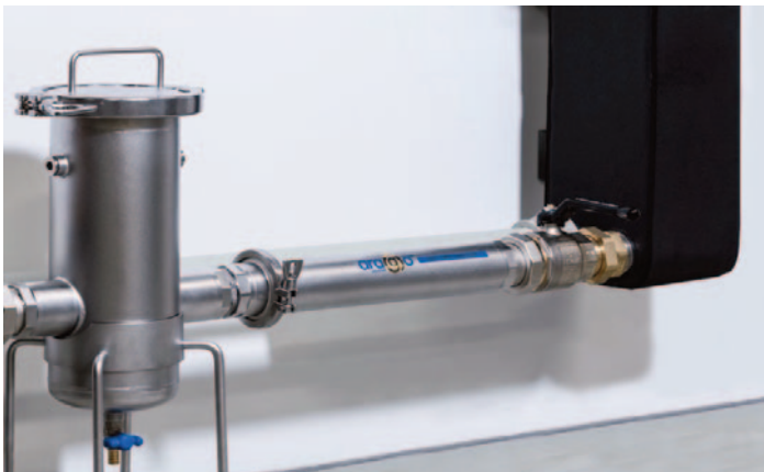
Example of Arago Industry water treatment plant and mechanical filter installation
